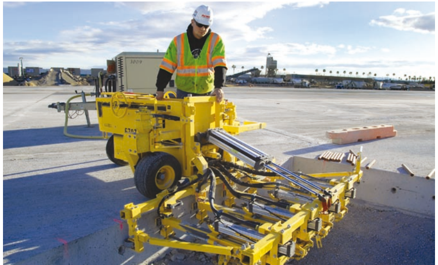
Pneumatic-powered concrete drills made it possible to drill the dowel bar holes without causing delays to the construction schedule. PHOTOS: ACME CONCRETE PAVING INC.
