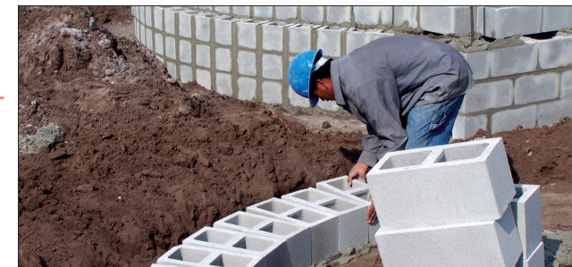
Right: The exterior walls combine autoclaved aerated concrete blocks that are filled with poured concrete. Photo: Robertson Homes
